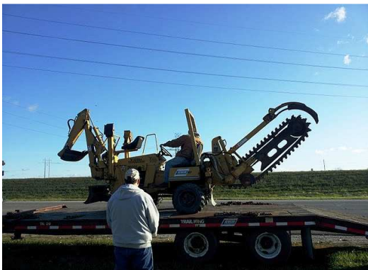
Ray Wiseman, back to camera, overseeing Tim Streit unloading a trencher provided by Newkirk Electric of Muskegon. The trencher is used to lay power lines at Muskegon's Veterans Memorial Park.
